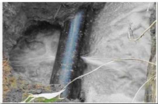
Figure. 2 Plastic pipe water leakages
