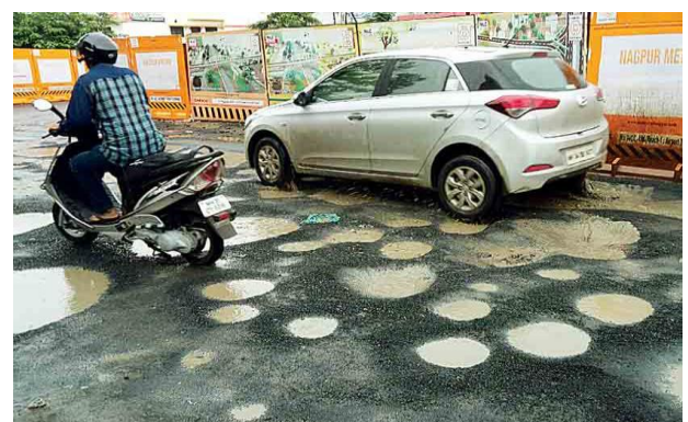
Fig. 1. Condition of roads with potholes
