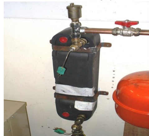
Figure 14. Shows the heat exchanger.
