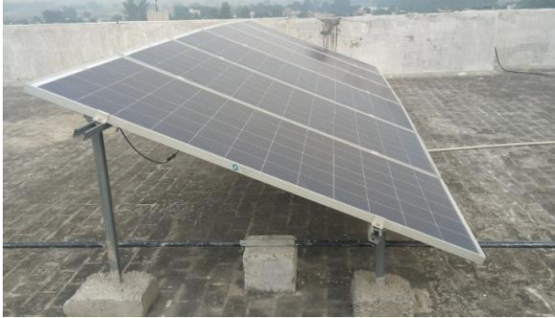
Fig 1. Top view of solar plant
