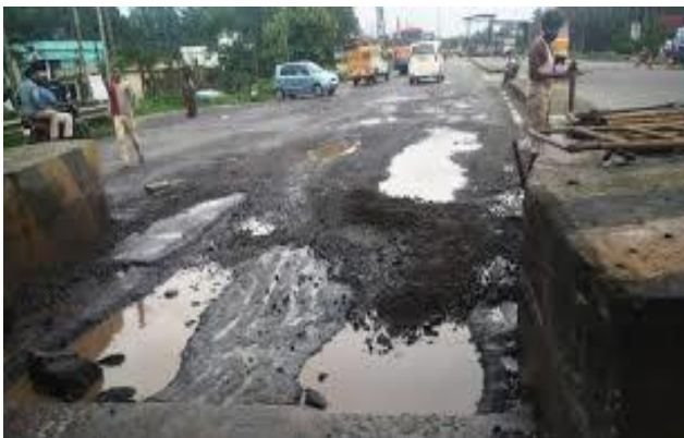
Figure 1 The Potholes and Road Damage
