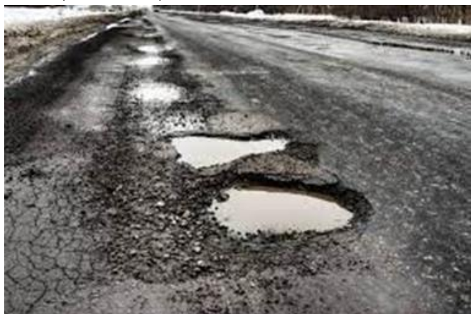
Fig. 1. Damaged roads surface with potholes.
