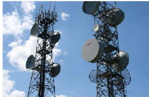
Figure 4. Cellular Transmission Towers.
