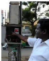
Operating street light manually
